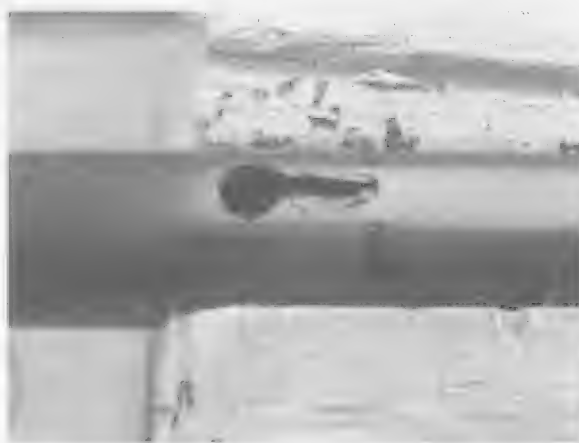
Figure 7-18 Hole and slot cut into electrical conduit.
